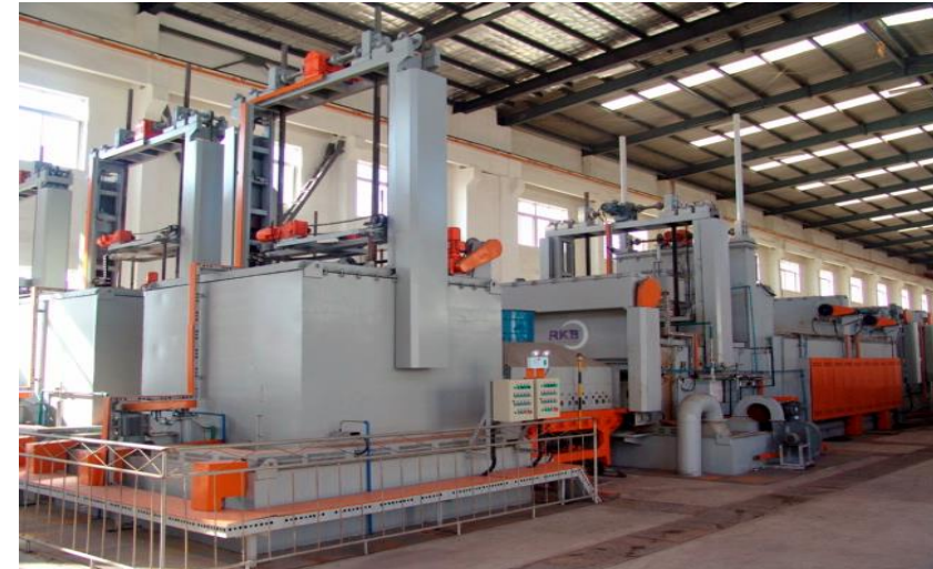
Furnaces for bainite treatment in RKB T3 Plant
